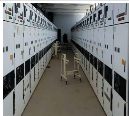
East Port Said Port Substation 220/22/22 kV Gas Insulated
